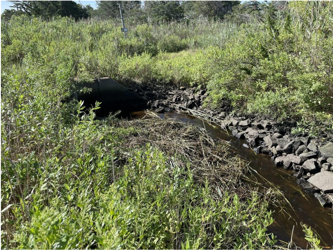
Photograph #3 – View of the western end of the work area where Common Reed has been removed.
